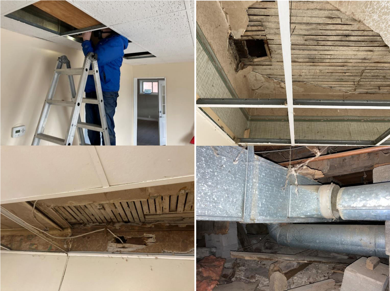
Above: Investigative work to uncover sources of air leakage, rodent ingress, and heat loss.
